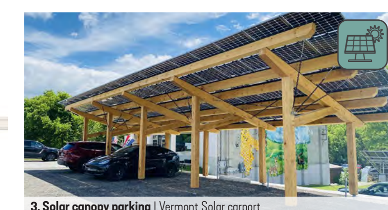
3. Solar canopy parking | Vermont Solar carport
